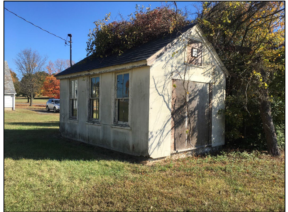
Photo 322: Building 1053, west and north elevations; photograph courtesy of Mark Edwards and Brian Clevon, 2016
