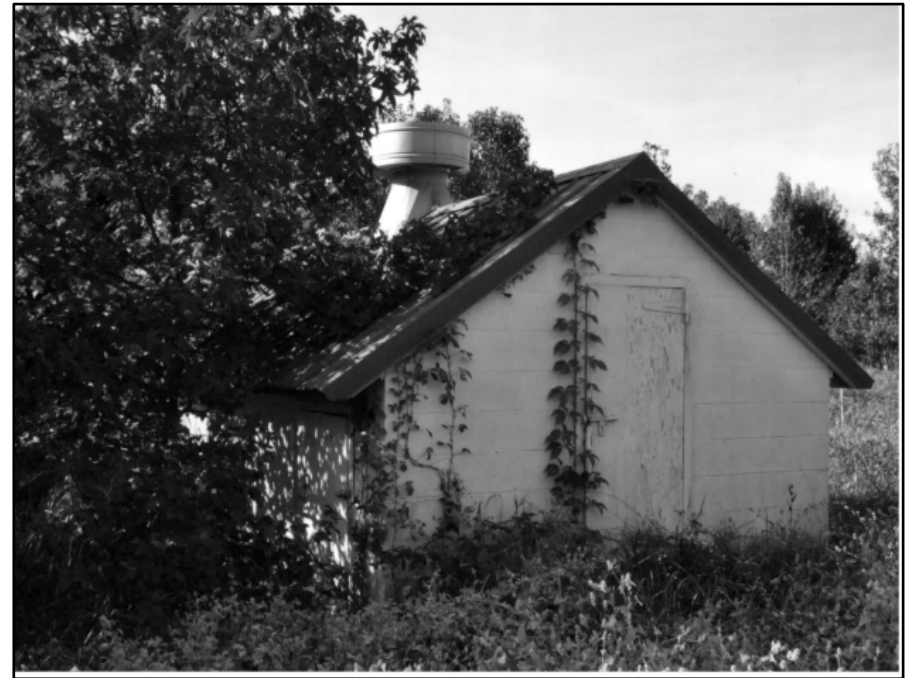
Photo 300: Building 0541D, east and north elevations; photograph courtesy of Mark Edwards and Brian Clevon, 2016
