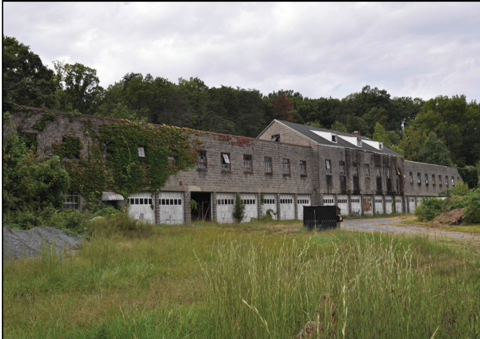
Photo 32: Building 0060, north elevation, camera facing southwest; photo courtesy of Mark Edwards and Brian Clevon, 2016
