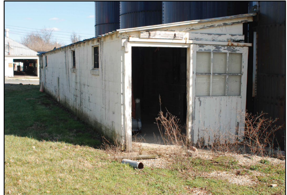
Photo 48: Building 0166A, north and west elevations; photograph courtesy of Mark Edwards and Brian Clevin, 2016
