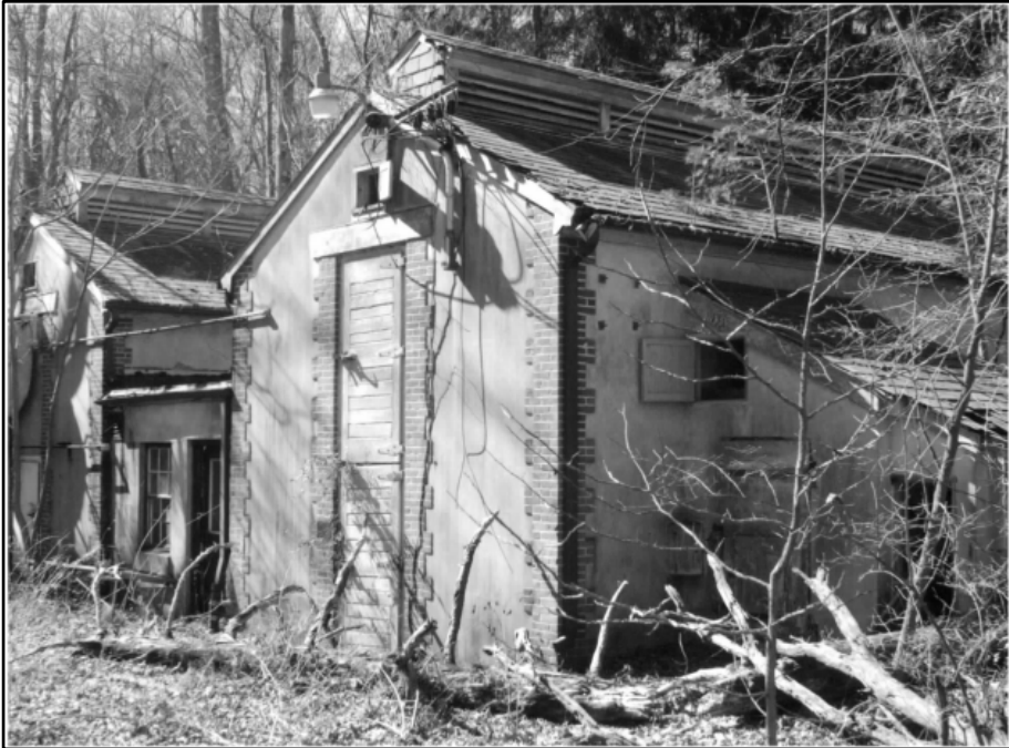
Photo 258: Building 0473, east and north elevations; photograph courtesy of Mark Edwards and Brian Clevon, 2016
