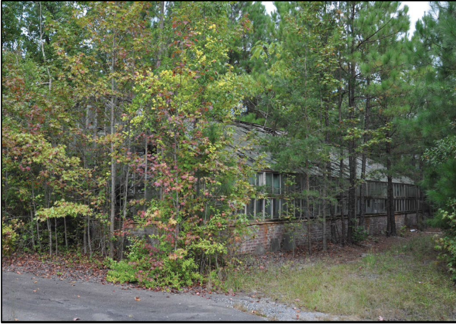
Photo 231: Building 0467, overview of south end of greenhouse; photograph courtesy of Brian Clevon, 2017
