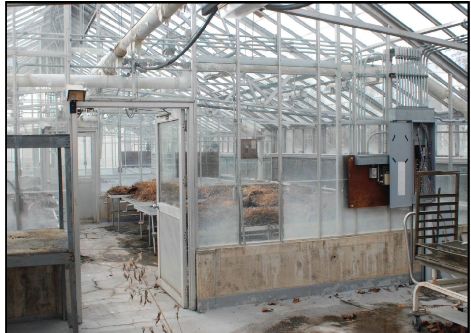
Photo 31: Building 0050, interior view of greenhouse; photograph courtesy of Mark Edwards and Brian Clevin, 2016
