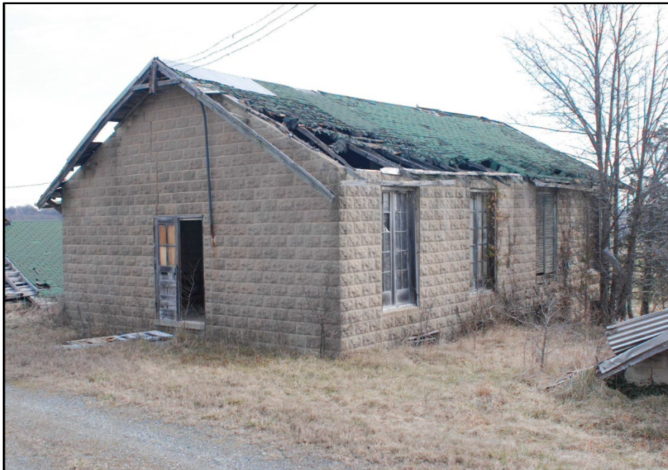
Photo 15: Building 0039, west and south elevations; photograph courtesy of Mark Edwards and Brian Clevin, 2016
