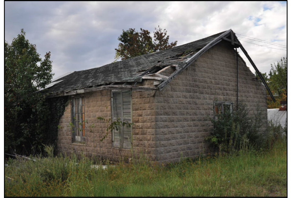
Photo 14: Building 0039, north and west elevations; photograph courtesy of Mark Edwards and Brian Clevin, 2016
