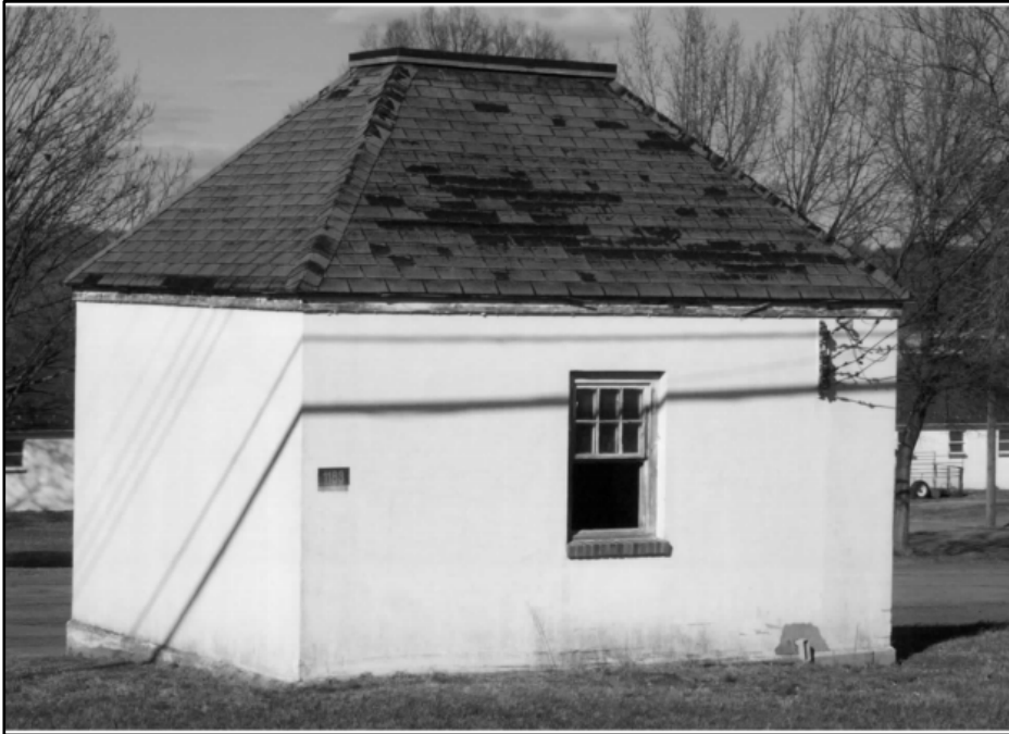
Photo 375: Building 1183, west and south elevations; photograph courtesy of Mark Edwards and Brian Clevon, 2016
